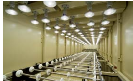
Interior of continuous process Class BBA production activation system
